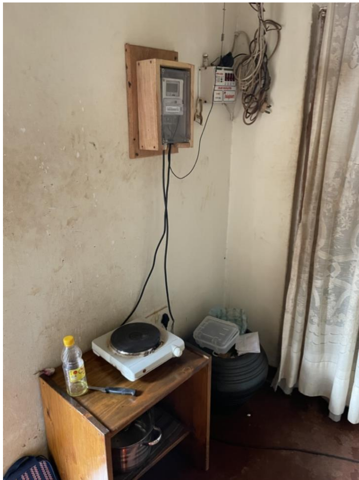
Figure 2: An electric cooking set installed in a pilot household
