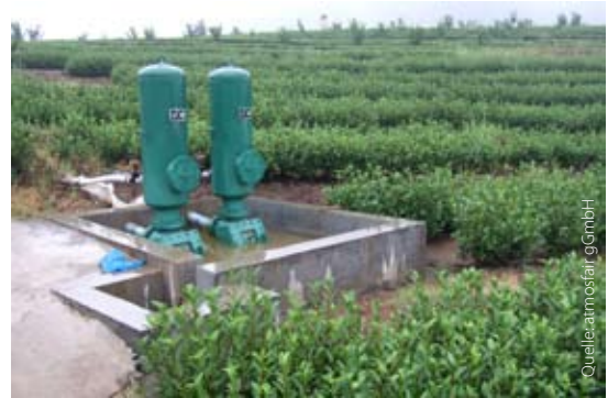
Irrigation system, China
