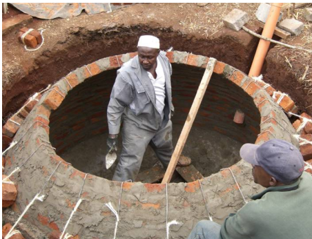
Biogas from cow dung (Kenya): The project supplies small biogas units to dairy farmers which produce regenerative biogas.
