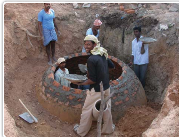
atmosfair project: Biogas units in India
