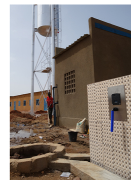
Core system with water tank, technical room for the water treatment plant and water dispenser station @atmosfair
