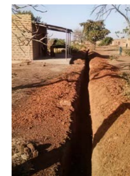
Laying the pipeline network and refilling water at another dispenser station in Dedougou @atmosfair
