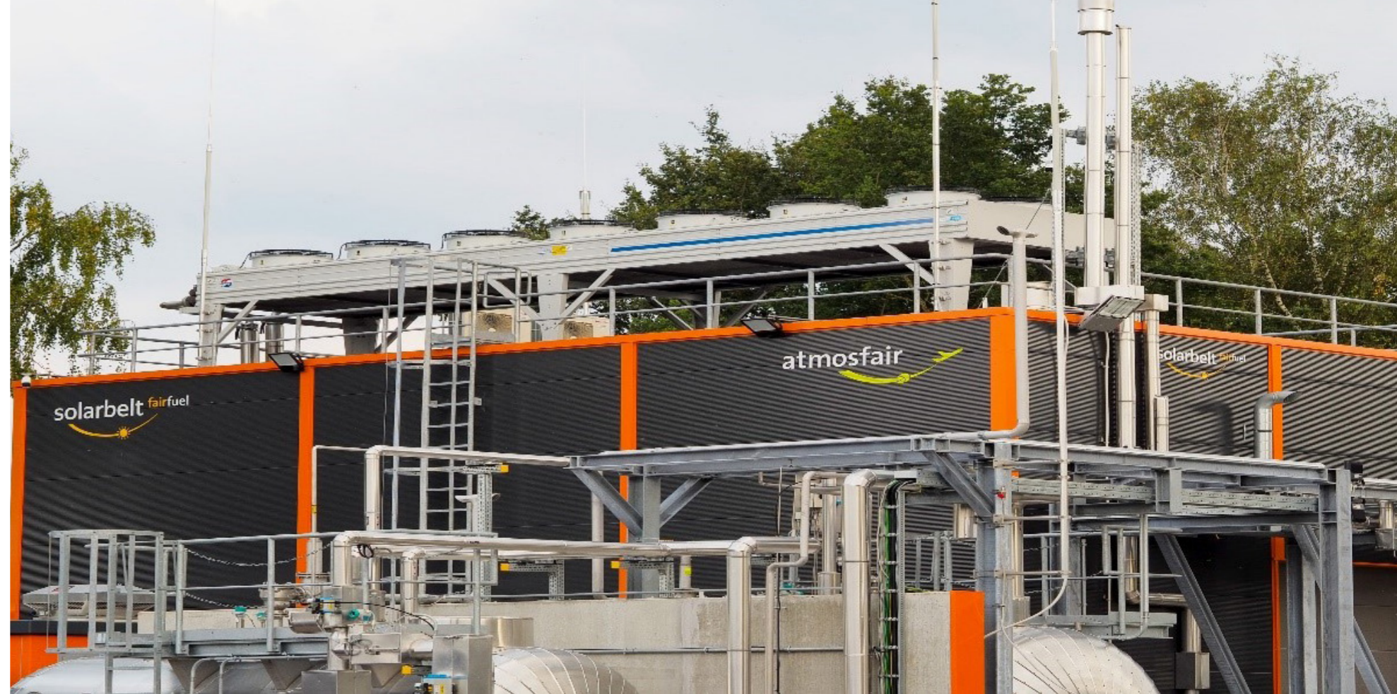
atmosfair e-kerosene plant in Werlte, October 2021
